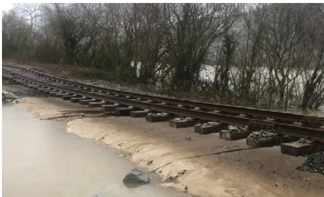
Conwy Valley railway line washed away by Storm Ciara, 2020
